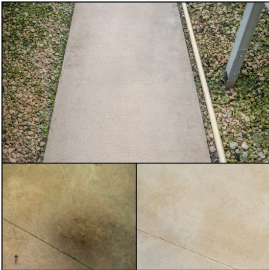
Pool shock and a broom on a prewetted surface cleaned up walkways, no slipping hazard!
